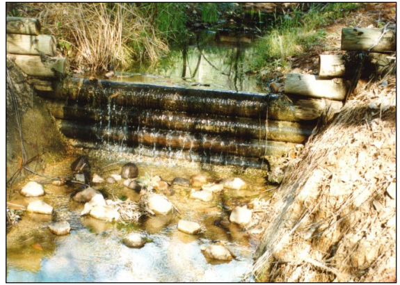
Picture 1: Major drop structure made of logs. Note the concrete and rock apron, and the concrete keying the logs into the side
