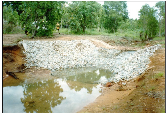
Picture 2: Major drop structure constructed from loose rock held in place by wire netting. Note stilling basin in the centre of the picture
