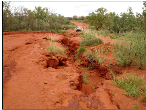
Picture 1: Poorly located roads directly up slope are prone to erosion
