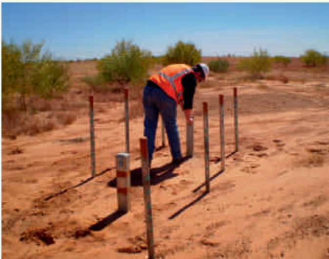
Independent Monitor Hydrogeologist, Geordie McMillan inspecting two new groundwater bores installed within the TSF Cell 1.
