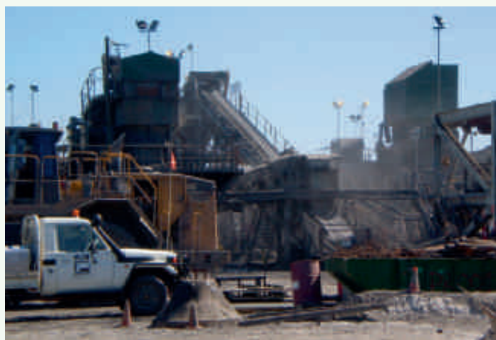
The 'PACRIM' ore crushing plant is the primary source of contaminated dust generated at the Mine site. Dust needs to be further reduced here.
