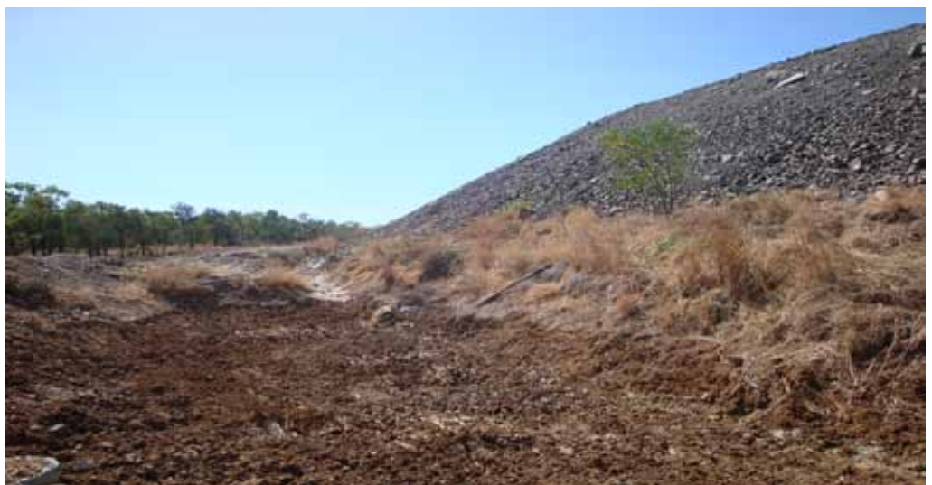
Failed drain and sump at the base of the Run of Mine Pad at the Mine site undergoing rehabilitation (Photo June 2009, Independent Monitor).
