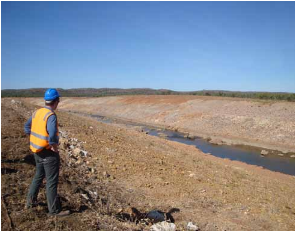
An Independent Monitor Team Member inspecting a section of the McArthur River diversion (Photo by Independent Monitor, June 2009)
