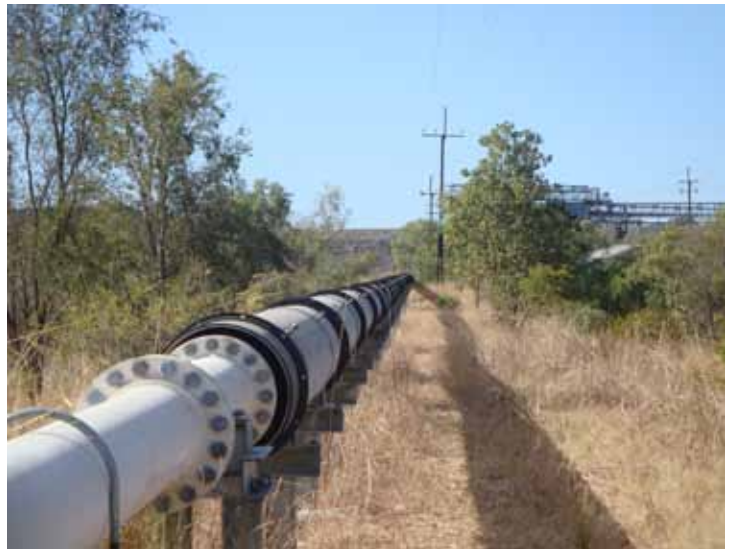
Pipeline that carries the tailings slurry from the processing plant to the Tailings Storage Facility (Photo June 2009, Independent Monitor).
