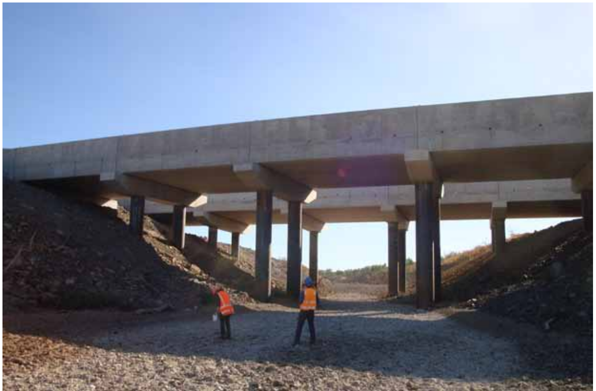
A portion of the Barney Creek diversion beneath the mine site bridge (Photo June 2009, Independent Monitor)
