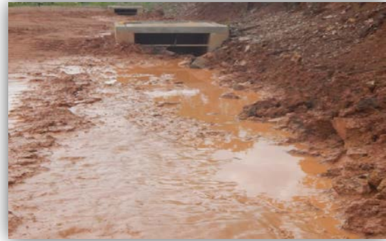
Onsite inlet pit - no sediment control protection
