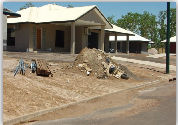
Un-managed soil & material stockpiles
