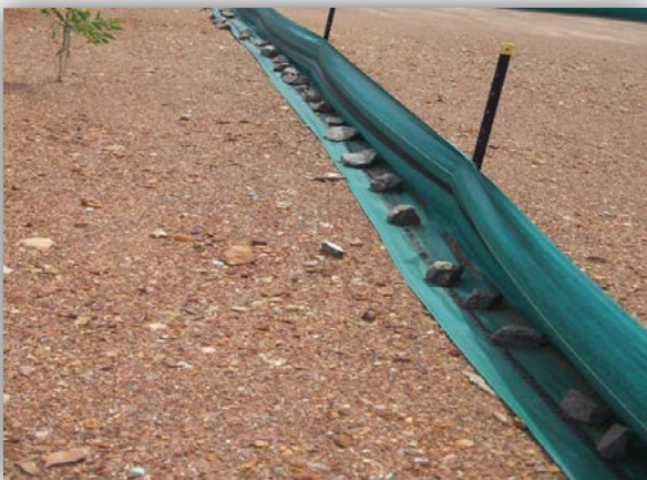
Sediment Fence- Not installed correctly
