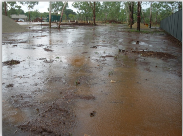
Construction site inaccessible after rain - lack of drainage and no diversion of upslope run-on.
