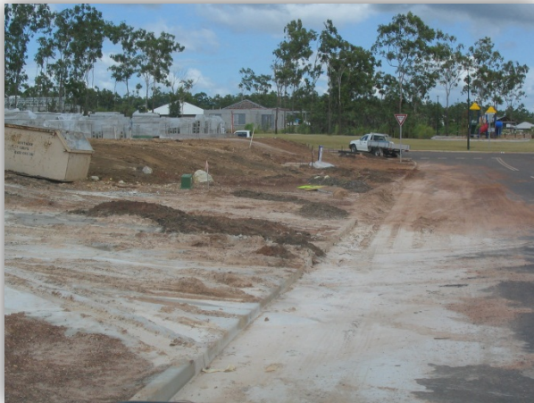
Uncontrolled site access, causing drainage to the verge and sediment discharge to the street, stormwater drainage system and local waterways.
