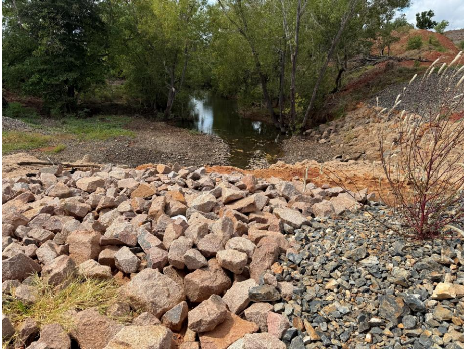
Plate 3 Erosion protection at the EBDC crossing appears to remain intact or has been appropriately repaired.
