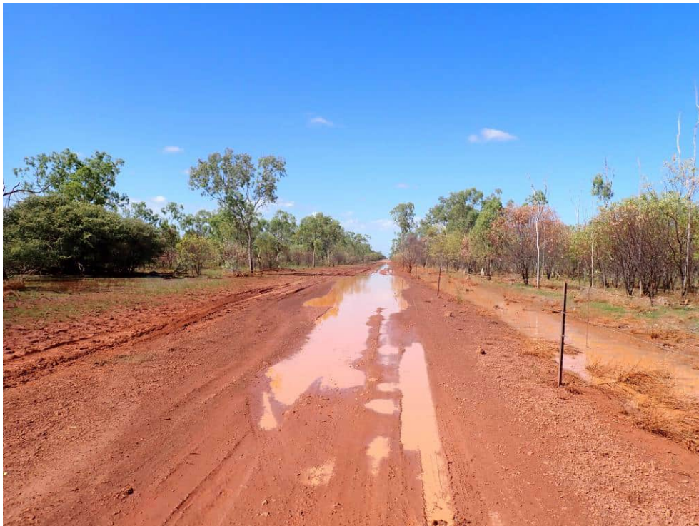
Figure 2.3 Example of ponded surface water, Photograph P5300235.JPG, Location A4 (see Figure 2.1)
