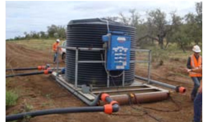
MRM have utilised a new irrigation sled to help establish vegetation along the McArthur River diversion channel over the 2010 dry season (May 2010).
