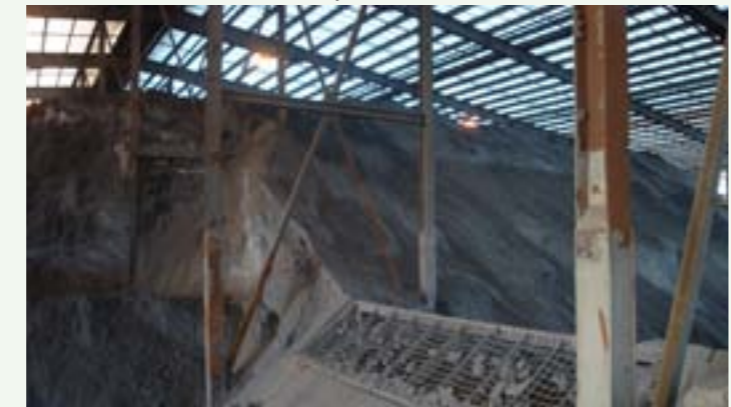
Zinc concentrate is stored within the Bing Bong concentrate storage shed while awaiting loadout onto the Arburri barge for shipment. The doors of the shed remain open to limit gas build-up that corrodes shed infrastructure. However, the open doors also allow concentrate dust to escape and spread via the wind to potentially contaminate soil, water or and sea sediments. This past year, damaged sections of the warehouse corrugated iron roof were replaced with fibreglass roofing that is resistant to the corrosive gases. The upgrade of the roof will assist in reducing dust emissions at the load out facility
