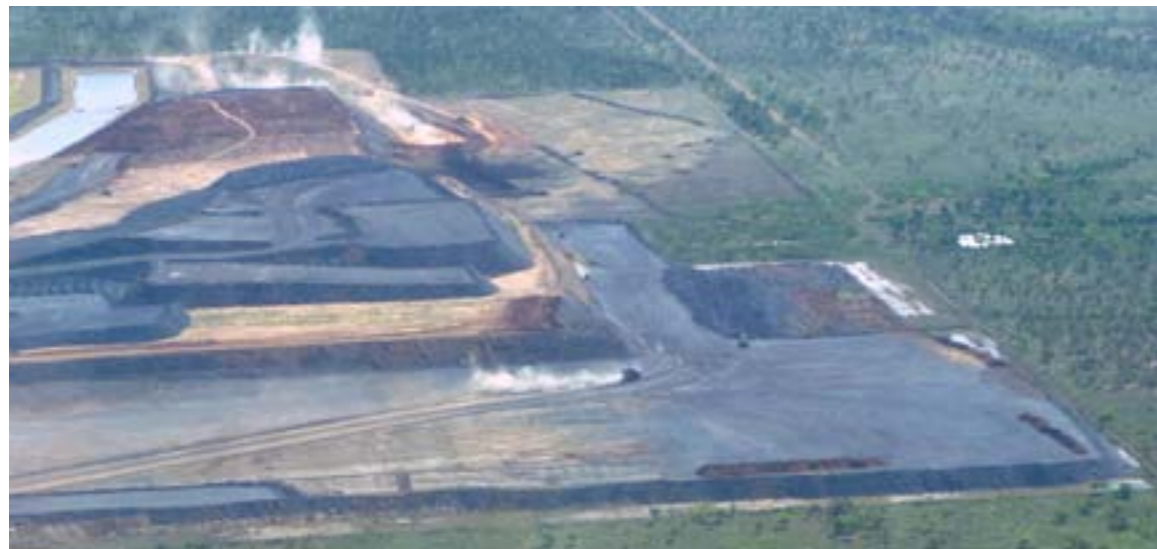
The clay layer that lines the base of the OEF is an essential part of the OEF design. The clay acts as a barrier to stop the migration of any acid production that may occur within the OEF waste rock. It is essential that the chemical and physical nature of the clay is tested before and after it is placed at the OEF to ensure its suitability. (May 2010).
