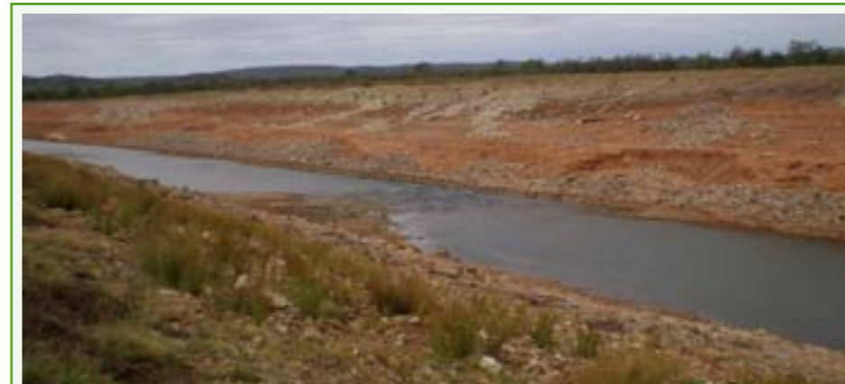
Minor slumping erosion and scour can be seen along the McArthur River diversion channel. Vegetation establishment, may help stabilise the banks of the diversion throughout the wet season floods. (May 2010)
